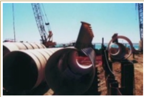
DN2200 GRP Offshore Cooling Water Pipework.
