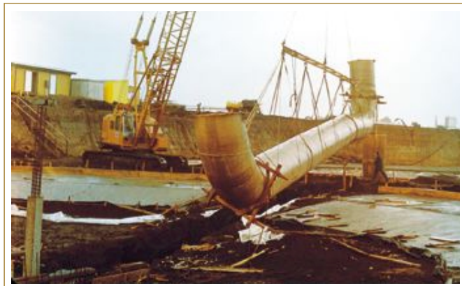
Inlet Pipe at Watercare Mangere, installed in 1978, still in service in 1999.
