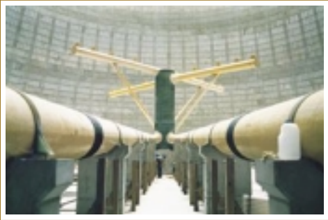
Hot gas diffuser structure inside cooling tower.
