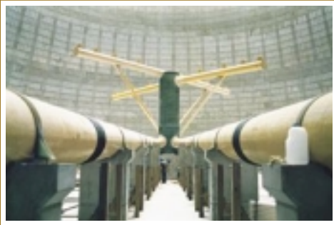
Hot gas diffuser structure inside cooling tower.
